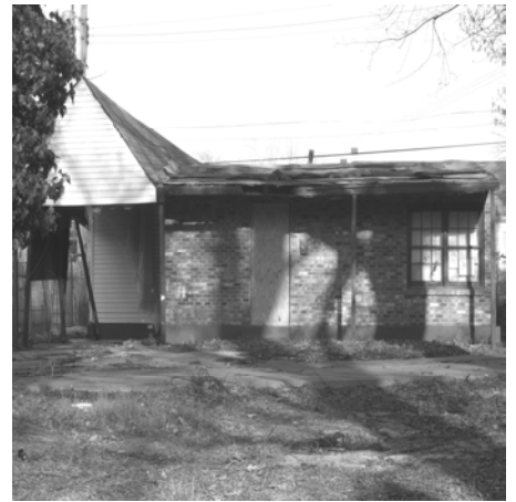
A severely damaged building at 1036 Maury that needs to be demolished by the City as soon as possible.
