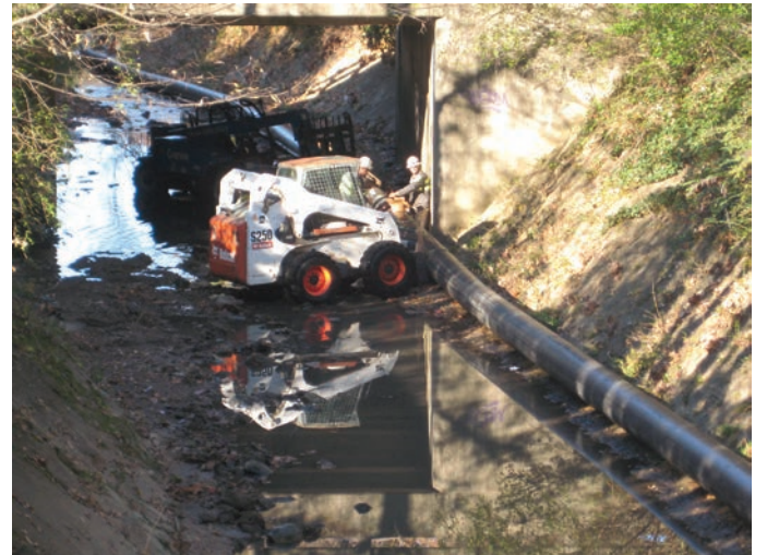
Above: Workers on Lick Creek working with the City of Memphis SARP10 (Sewer Assessment and Rehabilitation Program). Story on Page 11.
