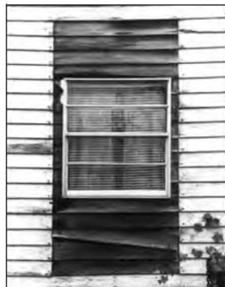
Image 84: The metal window is an obvious replacement for a much larger window that has been removed and the opening has been filled is not appropriate.
