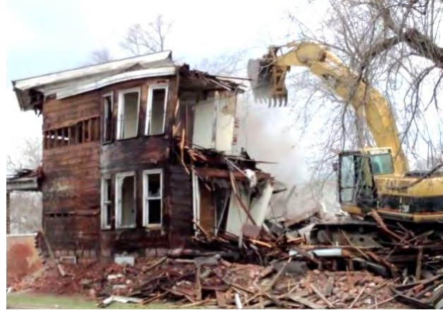
Image 88: (above) When demolition is the only alternative, salvage architectural historic elements for future reuse.
