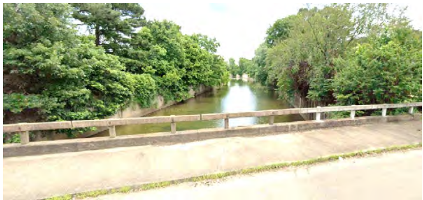
Image 79: (Above) Cypress Creek channelization project with concrete bridge railing along North McLean Boulevard.
