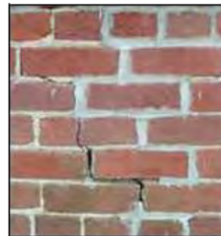
Image 83. The spot repointing of this wall does not match the original in color, texture, or form of joints. The dark gray color and texture of the mortar indicates that Portland cement mortar was used. The cracked and spalled brick (center top) resulted from the expansion of the harder Portland mortar.
